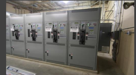
Power Distribution & Generation
