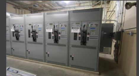
Power Distribution & Generation
