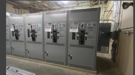
Power Distribution & Generation
