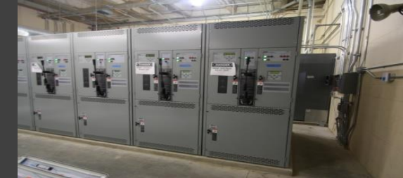
Power Distribution & Generation
