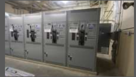
Power Distribution & Generation
