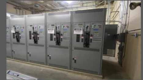
Power Distribution & Generation
